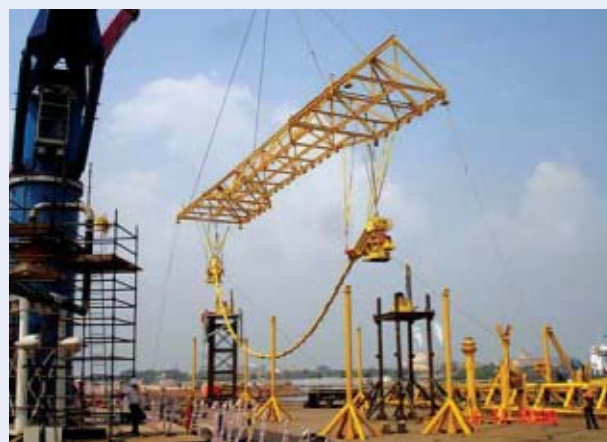
Bechtel oversaw fabrication, testing and system integration testing (SIT) of all jumpers onshore prior to offshore deployment.
